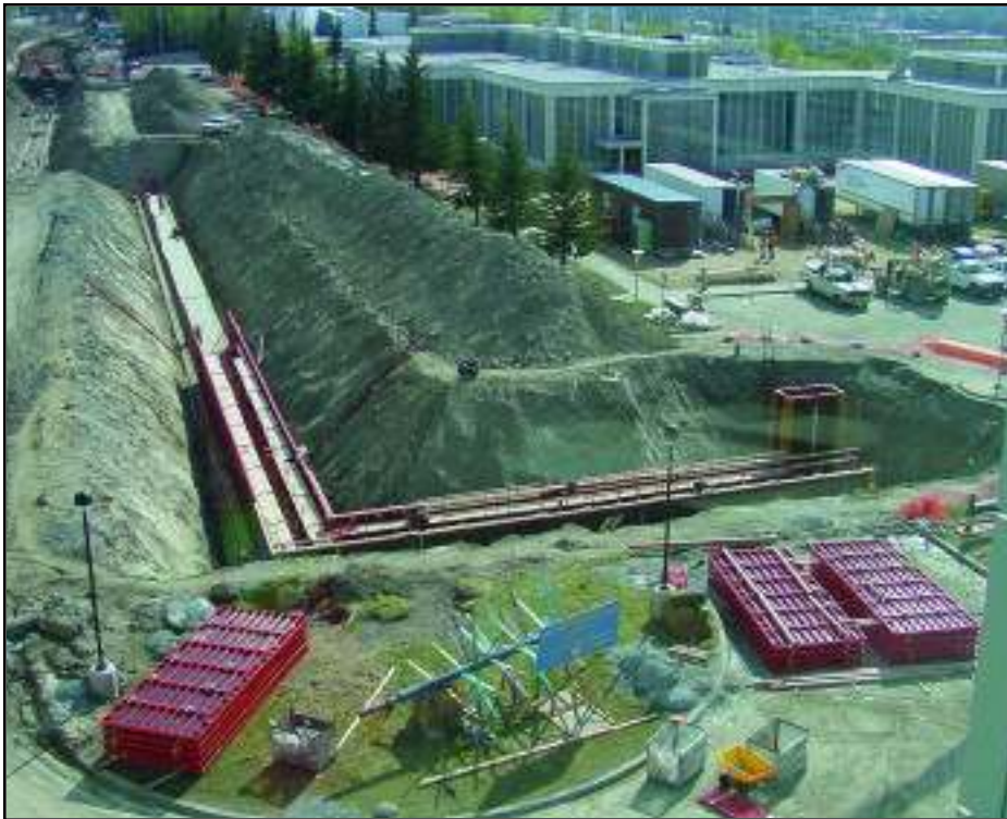
West Ridge Utilidor at UAF. With scientific research grants at UAF nearly doubling since 1977, new construction is booming.
