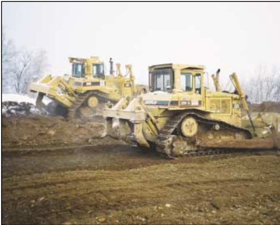
Tandem Caterpillar D-6 and D-9 dozers at NPI jobsite. Photo by Ron Arvin, Construction Manager, NPI, LLC.
