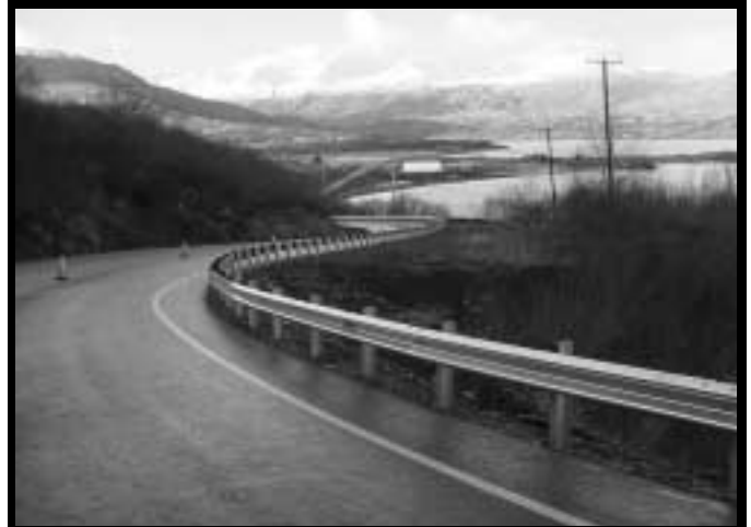
Acme Fence Company took the Ribelin Lowell Excellence in Construction Award for Kodiak Area Guardrail project.
