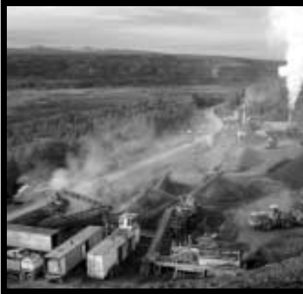
Winning top honors for transportation over $3 million was Wilder Construction for Elliot Highway MP28-72.
