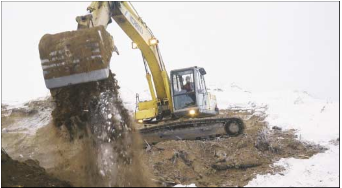
Operator working at NPI jobsite. Photo by Ron Arvin, Construction Manager, NPI, LLC.
