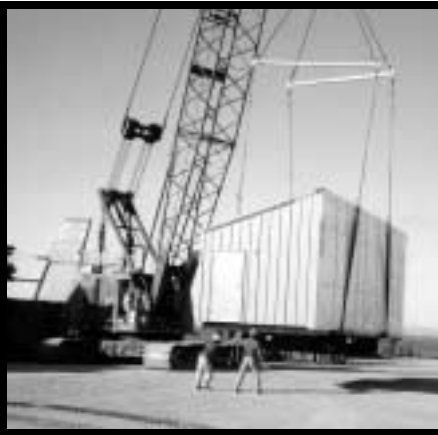
Alaska Modular won the specialty contractor award for vertical construction for Northwest Arctic Borough School District.
