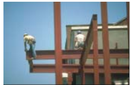
This worker is not protected by any of the protective systems that are required by OSHA.
