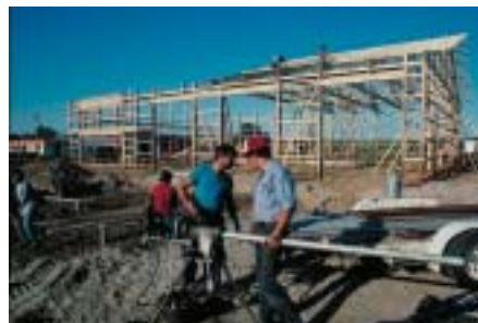
These workers are not protected from being struck by falling objects because they are working around/under other workers and not wearing hardhats.
