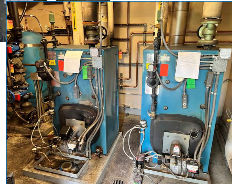
DFCS Juneau Johnson Youth Center Boiler Replacements
